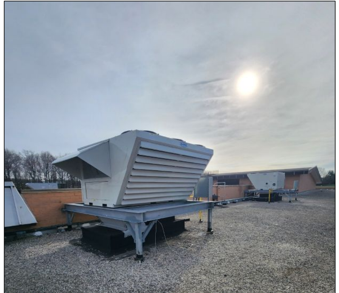
RTU #2 and #4 Installed & Started Up
