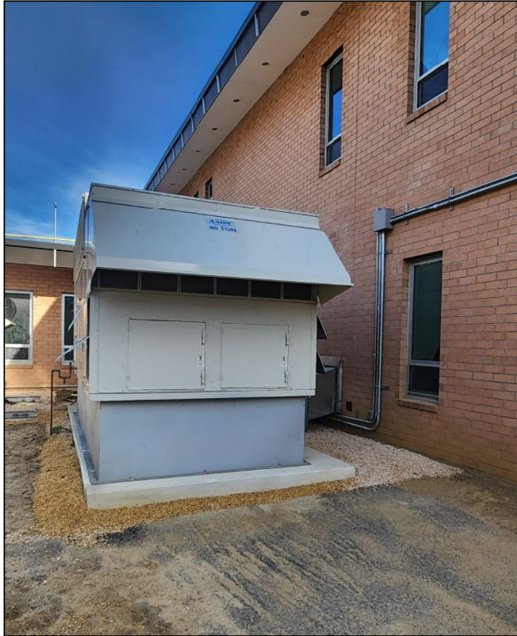
DOAS #1 Installed & Started Up
