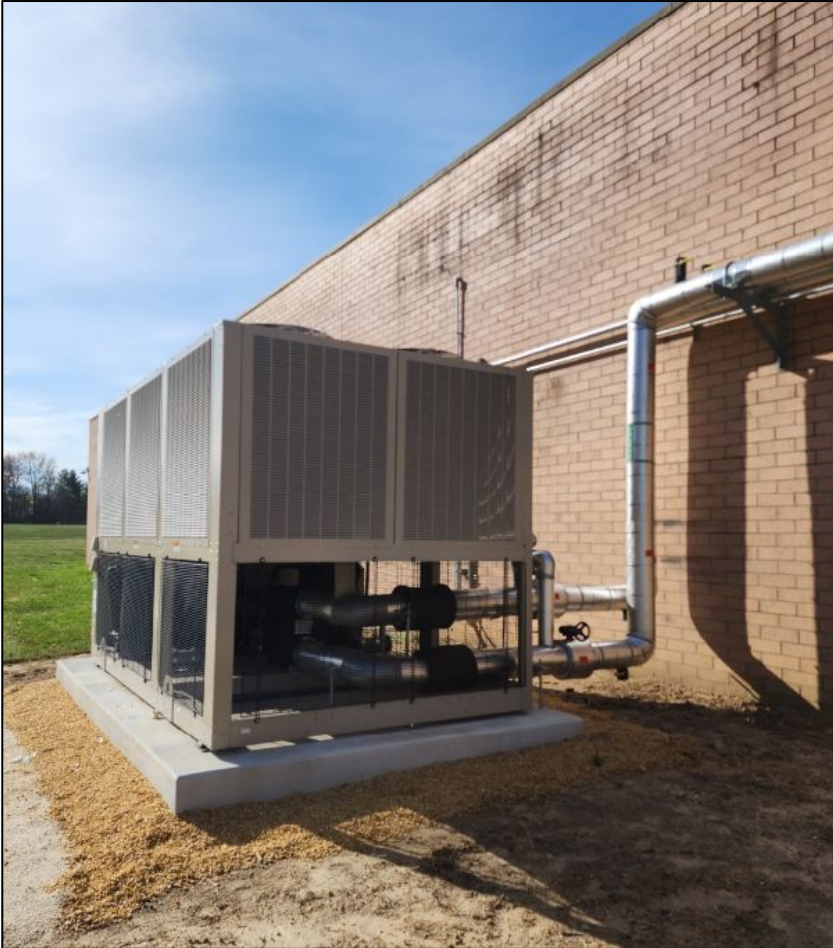
Chiller Installed & Started Up
