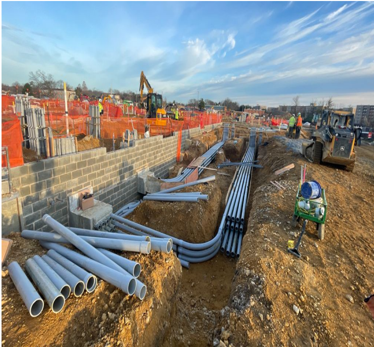
Incoming Electrical Duct Bank
