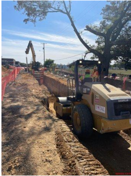
Soil compaction from manhole (MH) 2 to the middle of the west connector road.
