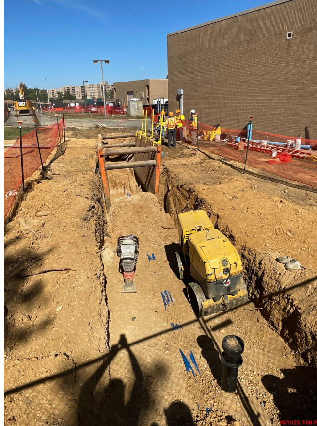
Soil compaction on top of the water line.
